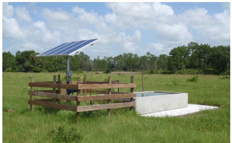
Alternative water source is a water quality best management practice that provides fresh water and limits the congregation of livestock in nearby streams and canals.
